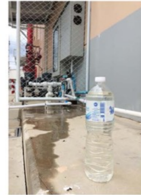
Effluent from MBR Tank
