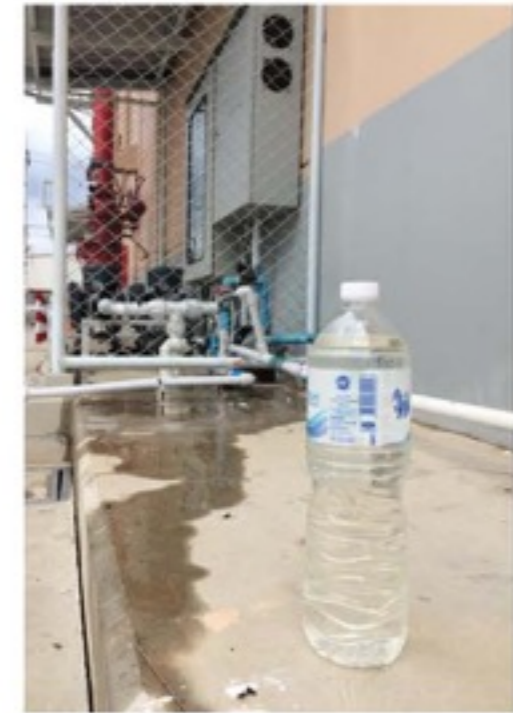
Effluent from MBR Tank
